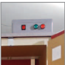
Control unit with fire detection
